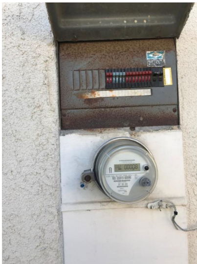
Old Meter Panel
