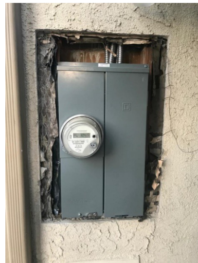
New Meter Panel prior to finishing framing
