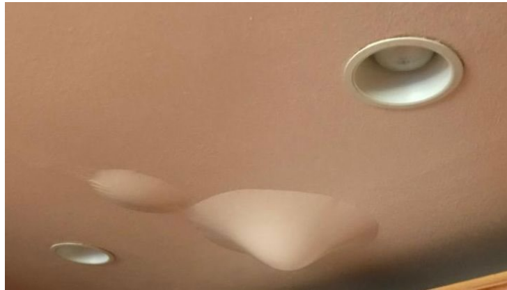
Caused this to the ceiling of the unit below
