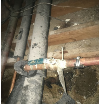
Leak in attic
