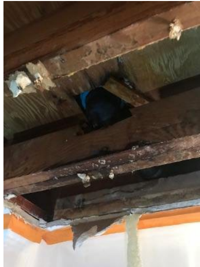
Damage recently occurring
