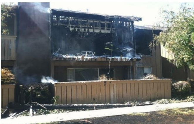
This charred townhouse embodies the worries driving Grill bans: An Unattended grill displaced nine people In Hayward, California. Source: CBS SP BayArea
