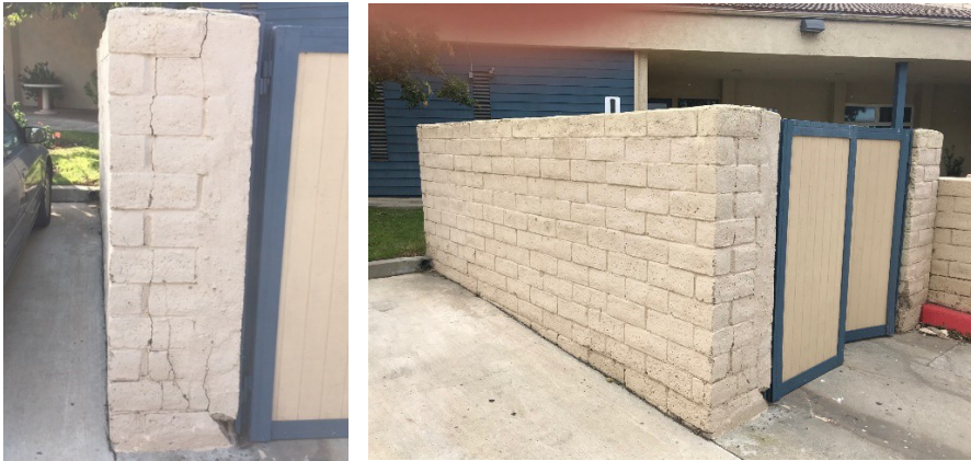
Damaged trash enclosure
