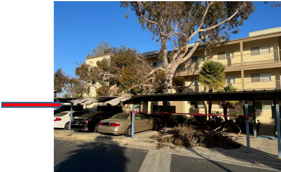
Damaged Building 5 Carport
