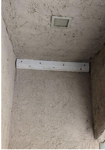
3rd floor end of building with the reinforcement at the high ceiling
