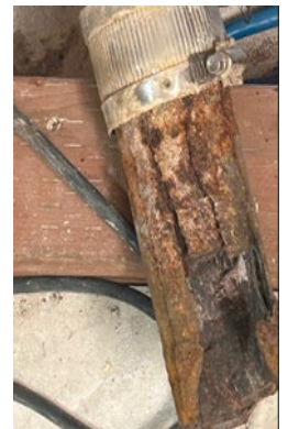
Tub drainpipe that caused damage due to leaking water.
