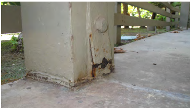
4. ORIGINAL - 8/10/21 (ELEVATED WALK- RUST AT HARDWARE)
