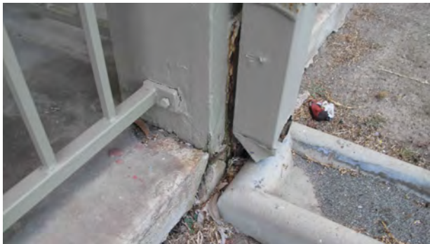
4. ORIGINAL - 8/10/21 (ELEVATED WALK- RUST AT HARDWARE)
