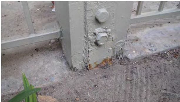
6. ORIGINAL - 8/10/21 (ELEVATED WALK- RUST AT HARDWARE)
