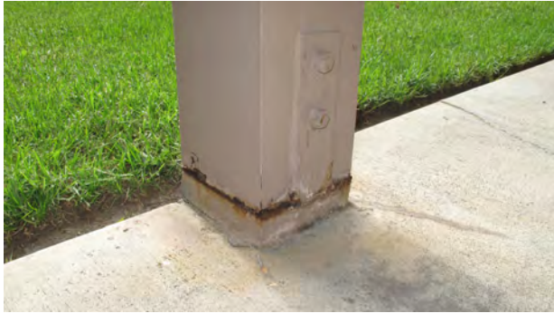
5. ORIGINAL - 8/10/21 (ELEVATED WALK- RUST AT HARDWARE)
