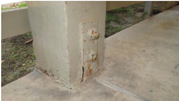
8. ORIGINAL - 8/10/21 (ELEVATED WALK- RUST AT HARDWARE)
