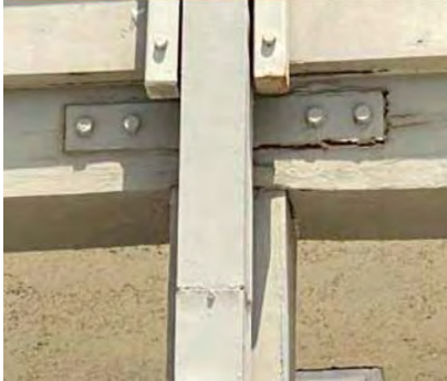
A. ORIGINAL - 8/10/21 (UNIT 643 - DRY ROT AT BEAM)
