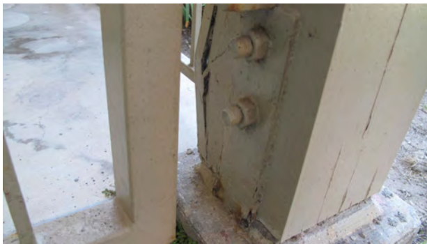
3. ORIGINAL - 8/10/21 (ELEVATED WALK- RUST AT HARDWARE)
