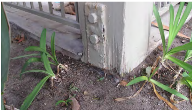
7. ORIGINAL - 8/10/21 (ELEVATED WALK- RUST AT HARDWARE)
