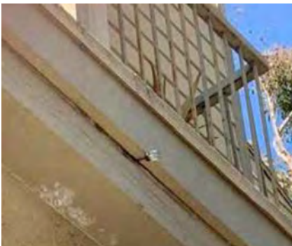
C. ORIGINAL - 8/10/21 (UNIT 576 - DRY ROT AT BEAM)
