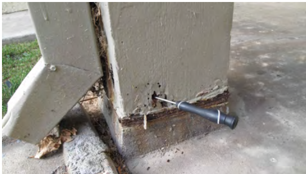
2. ORIGINAL - 8/10/20212. (ELEVATED WALK- DRY ROT AT POST)
