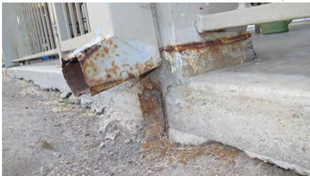
4. ORIGINAL - 8/10/21 (ELEVATED WALK- RUST AT HARDWARE)
