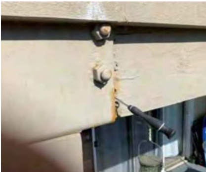
B. ORIGINAL - 8/10/21 (UNIT 570 - DRY ROT AT BEAM)
