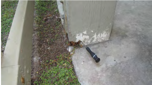
5. ORIGINAL - 8/10/21 (ELEVATED WALK- DRY ROT AT POST)
