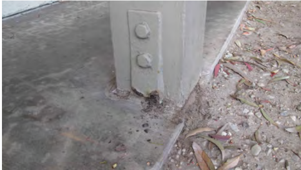
1. ORIGINAL - 8/10/21 (ELEVATED WALK- RUST AT HARDWARE)
