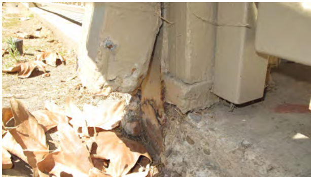
2. ORIGINAL - 8/10/21 (ELEVATED WALK- RUST AT HARDWARE)
