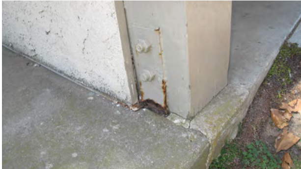
1. ORIGINAL - 8/10/21 (ELEVATED WALK- RUST AT HARDWARE)
