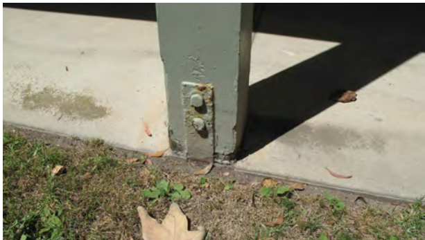
2. ORIGINAL - 8/10/21 (ELEVATED WALK- RUST AT HARDWARE)
