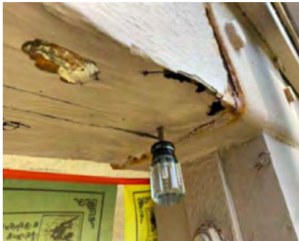
A. ORIGINAL - 8/10/21 (UNIT 616 - DRY ROT AT BEAM)
