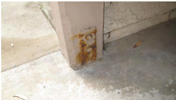
4. ORIGINAL - 8/10/21 (ELEVATED WALK- RUST AT HARDWARE)
