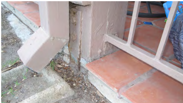
10. ORIGINAL - 8/10/21 (ELEVATED WALK- RUST AT HARDWARE)
