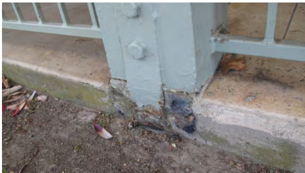
4. ORIGINAL - 8/10/21 (ELEVATED WALK- RUST AT HARDWARE)
