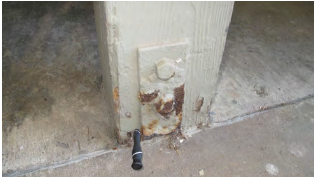
1. ORIGINAL - 8/10/21 (ELEVATED WALK- DRY ROT AT POST AND RUST AT HARDWARE)
