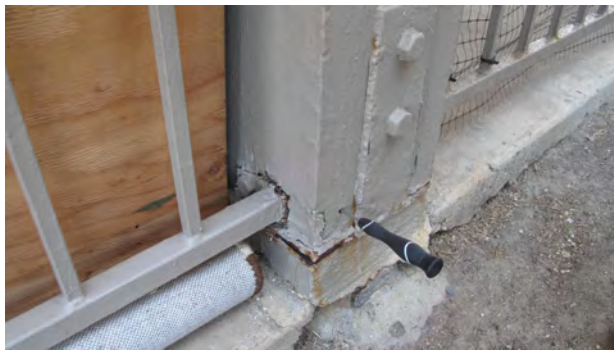
7. ORIGINAL - 8/10/21 (ELEVATED WALK- DRY ROT AT POST AND RUST AT HARDWARE)
