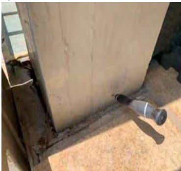
B. ORIGINAL - 8/10/21 (UNIT 685 - DRY ROT AT BEAM)
