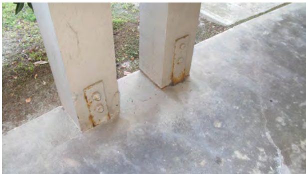
4. ORIGINAL - 8/10/21 (ELEVATED WALK- RUST AT HARDWARE)
