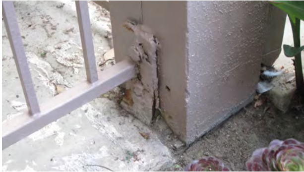
1. ORIGINAL - 8/10/21 (ELEVATED WALK- RUST AT HARDWARE)
