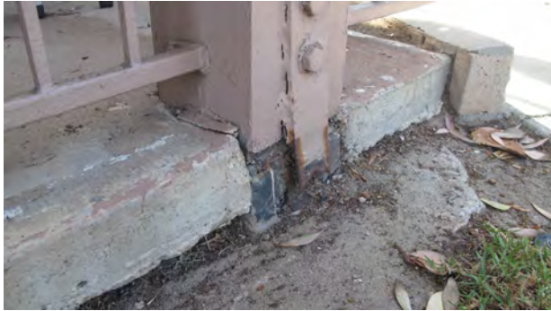
13. ORIGINAL - 8/10/21 (ELEVATED WALK- RUST AT HARDWARE)
