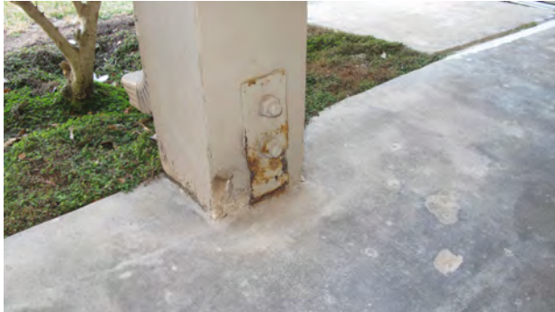
1. ORIGINAL - 8/10/21 (ELEVATED WALK- RUST AT HARDWARE)
