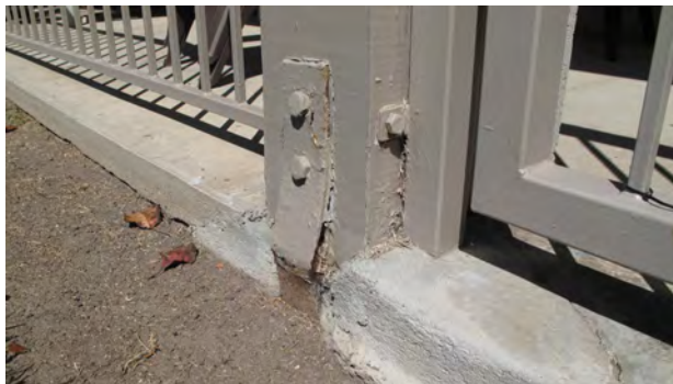
8. ORIGINAL - 8/10/21 (ELEVATED WALK- RUST AT HARDWARE)
