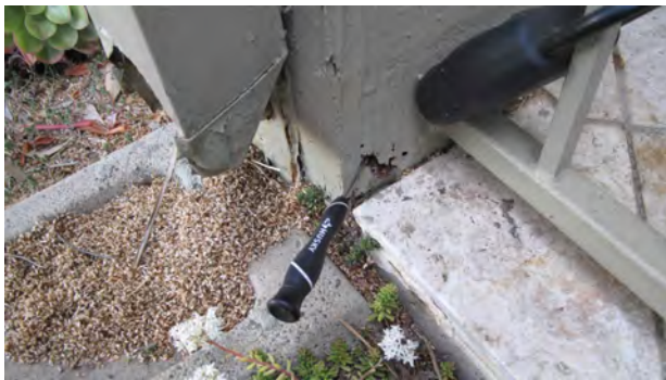
3. ORIGINAL - 8/10/21 (ELEVATED WALK- DRY ROT AT POST)
