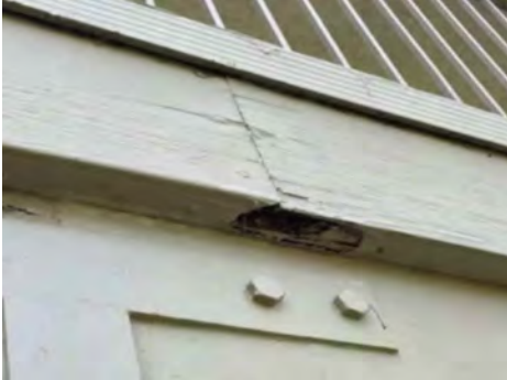
A. ORIGINAL - 8/10/21 (ELEVATED WALK WAY - DRY ROT AT POST/BEAM)
