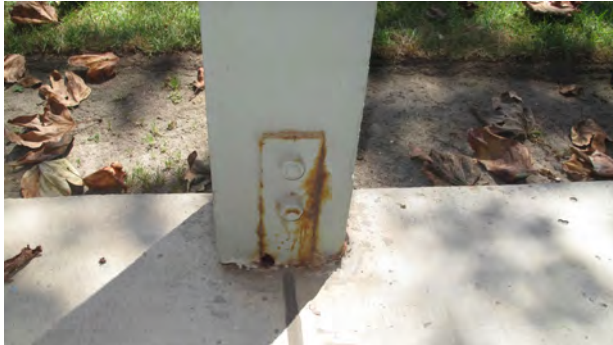
1. ORIGINAL - 8/10/21 (ELEVATED WALK- RUST AT HARDWARE)
