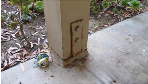
1. ORIGINAL - 8/10/21 (ELEVATED WALK- RUST AT HARDWARE)
