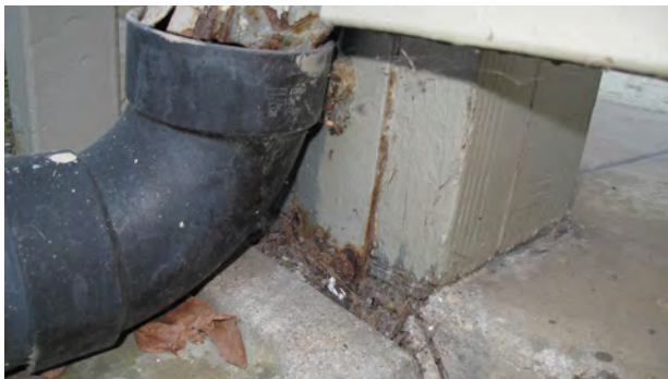
7. ORIGINAL - 8/10/21 (ELEVATED WALK- RUST AT HARDWARE)
