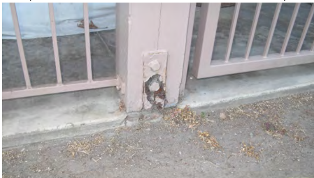
8. ORIGINAL - 8/10/21 (ELEVATED WALK- RUST AT HARDWARE)
