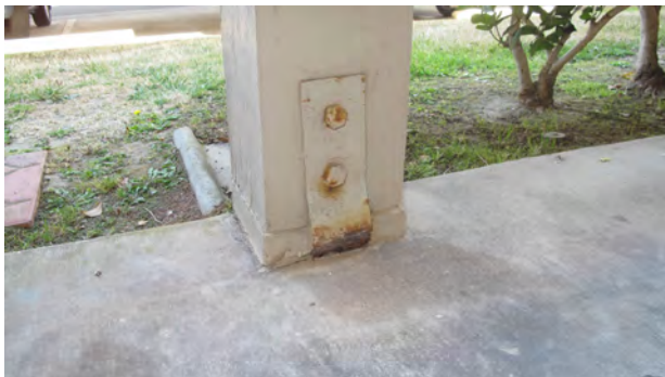
3. ORIGINAL - 8/10/21 (ELEVATED WALK- RUST AT HARDWARE)
