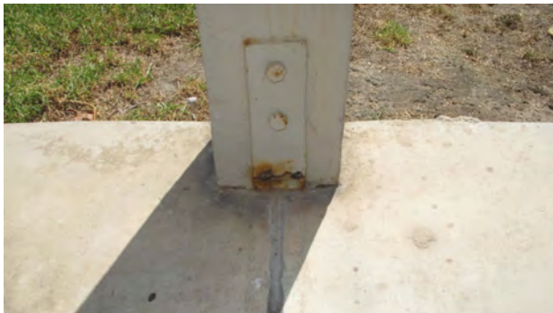
2. ORIGINAL - 8/10/21 (ELEVATED WALK- RUST AT HARDWARE)
