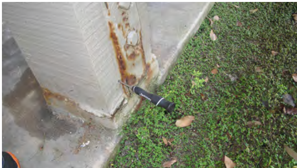
2. ORIGINAL - 8/10/21 (ELEVATED WALK- RUST AT HARDWARE AND DRY ROT AT POST)
