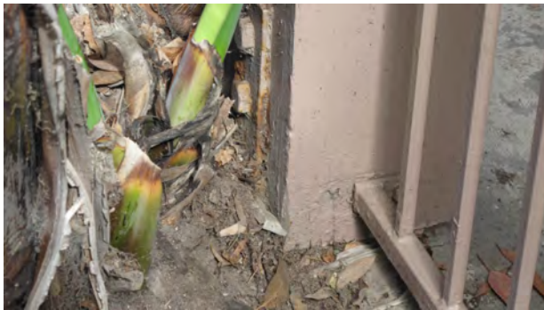
2. ORIGINAL - 8/10/21 (ELEVATED WALK- RUST AT HARDWARE)
