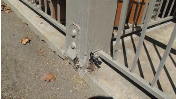
9. ORIGINAL - 8/10/21 (ELEVATED WALK- DRY ROT AT POST AND RUST AT HARDWARE)
