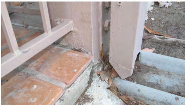
11. ORIGINAL - 8/10/21 (ELEVATED WALK- RUST AT HARDWARE)
