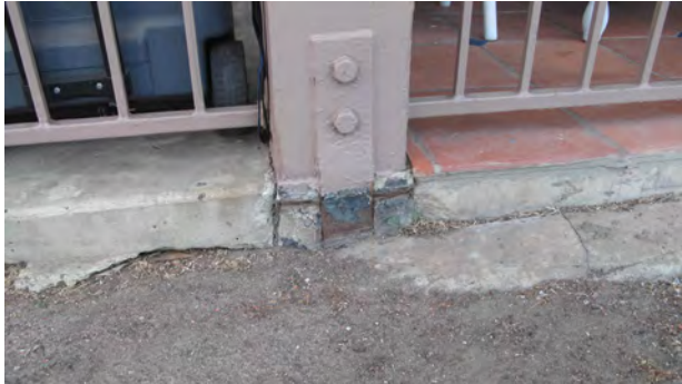
9. ORIGINAL - 8/10/21 (ELEVATED WALK - RUST AT HARDWARE)
