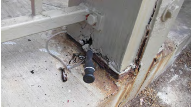
5. ORIGINAL - 8/10/21 (ELEVATED WALK- DRY ROT AT POST)
