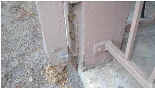
7. ORIGINAL - 8/10/21 (ELEVATED WALK- RUST AT HARDWARE)
