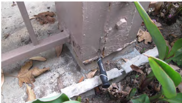
3. ORIGINAL - 8/10/21 (ELEVATED WALK- RUST AT HARDWARE AND DRY ROT AT POST)
