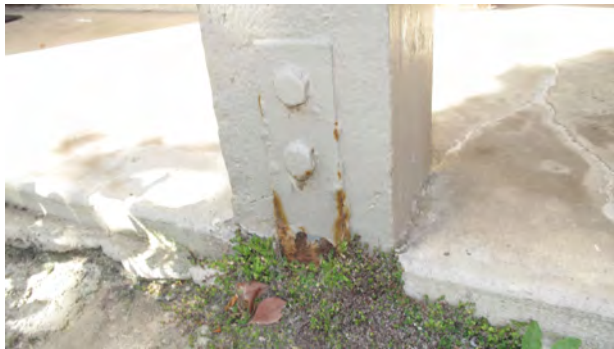
6. ORIGINAL - 8/10/21 (ELEVATED WALK- RUST AT HARDWARE)
