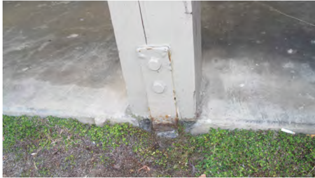
5. ORIGINAL - 8/10/21 (ELEVATED WALK- RUST AT HARDWARE)
