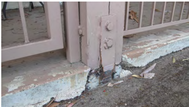
12. ORIGINAL - 8/10/21 (ELEVATED WALK- RUST AT HARDWARE)
