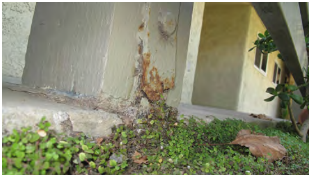
6. ORIGINAL - 8/10/21 (ELEVATED WALK- RUST AT HARDWARE)
