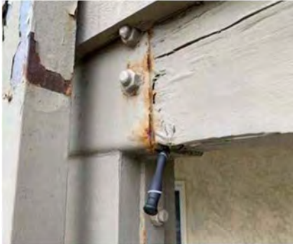
A. ORIGINAL - 8/10/21 (UNIT 512 - DRY ROT AT BEAM)
