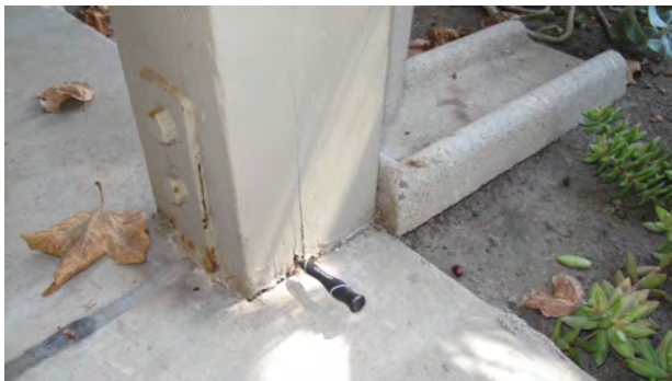
3. ORIGINAL - 8/10/21 (ELEVATED WALK- DRY ROT AT POST AND RUST AT HARDWARE)
