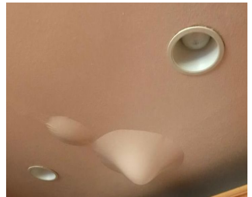
Sample 1 st floor ceiling damage
