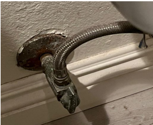
2 nd floor water valve
